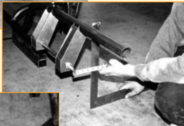
The lower A-arm brackets are attached to the Chassisworks assembly fixture and tacked to the frame rail as specified in the instructions. (This fixture not only assures correct spacing and alignment of both upper and lower brackets, but, after assembly, it can be returned undamaged to Chassisworks for a 50-percent refund.)
