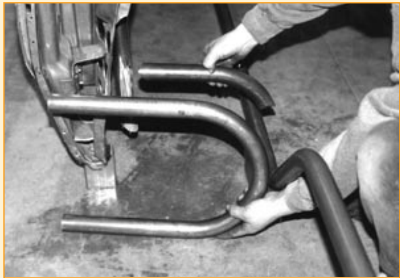
After the frame rails are in the car, they must be attached to the roll cage. Shown here is the Chassisworks cage-side-extension loop, which is cut in half to yield a brace for each side. The rise in the tubing allows for maximum header clearance under the car.
